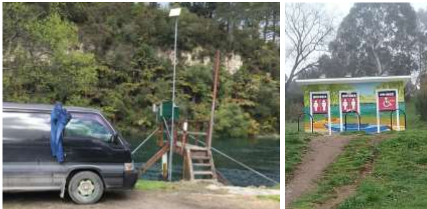
Figure 2: Water monitoring and toilet structures at Reid's farm
