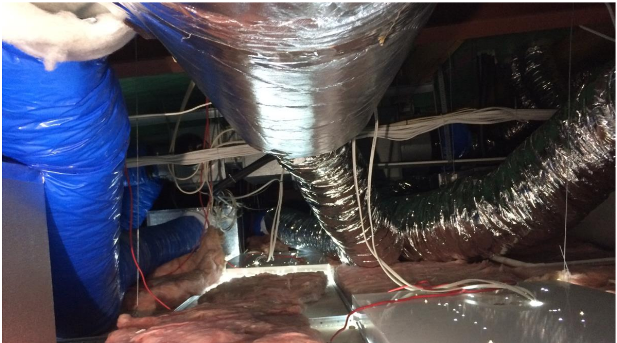
Redundant ducting and loose wiring can cause a fire hazard.
