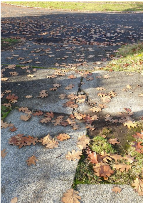
Above: Footpath break adjoining vehicle crossing Note vehicle scrape point where driveway meets path
