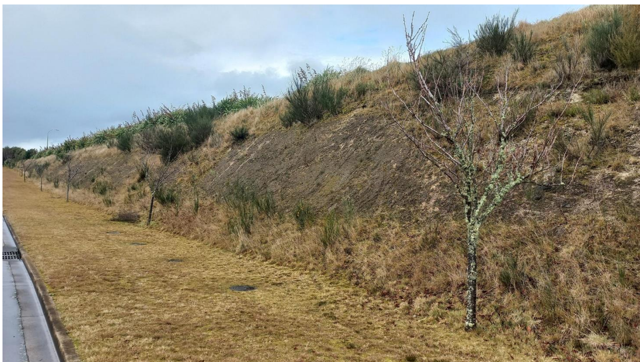
Image 5 – the poor state of Pukenuamu Road batters, showing 17 years of tree growth, bare banks and weed growth.
