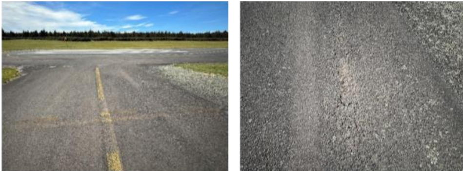
Figure 3-7: Taxiway A (N) - Accelerated weathering, aggregate loss
