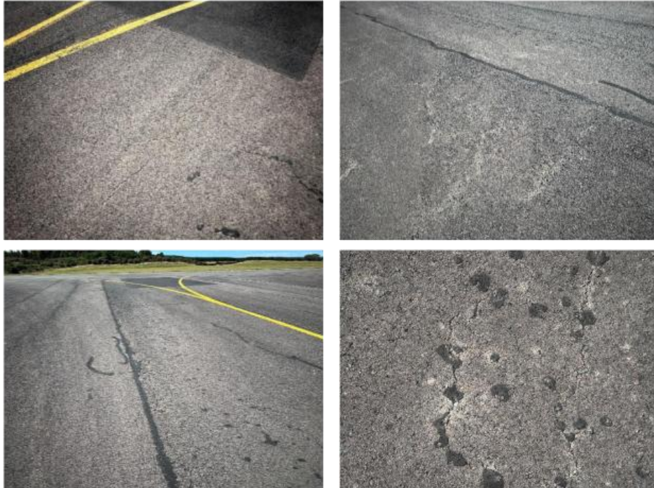
Figure 3-10: Taxiway B – Cracking, weathering, bleeding
