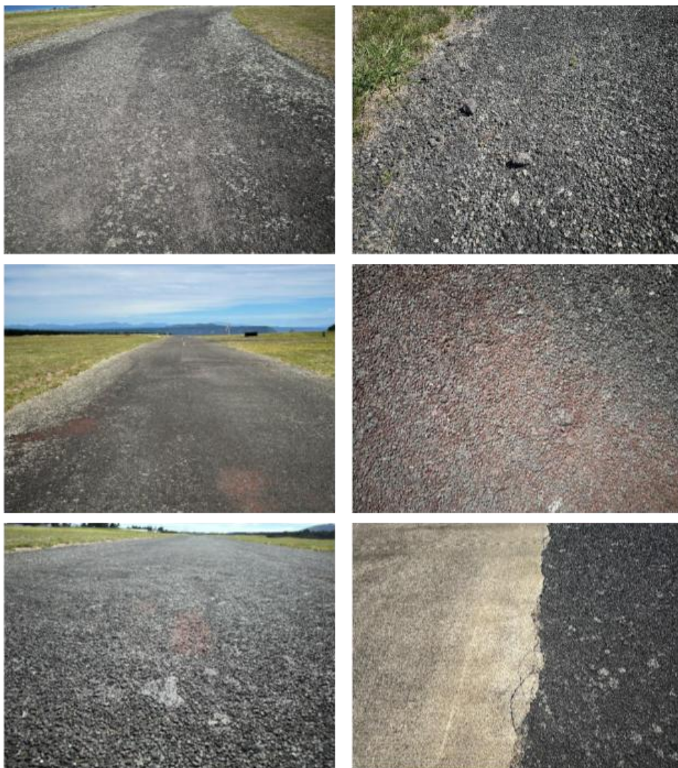
Figure 3-13: Taxiway E – Loose aggregate, red algae, Lichen
