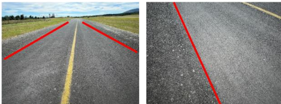
Figure 3-9: Taxiway A (widening) – Debonding, lichen growth
