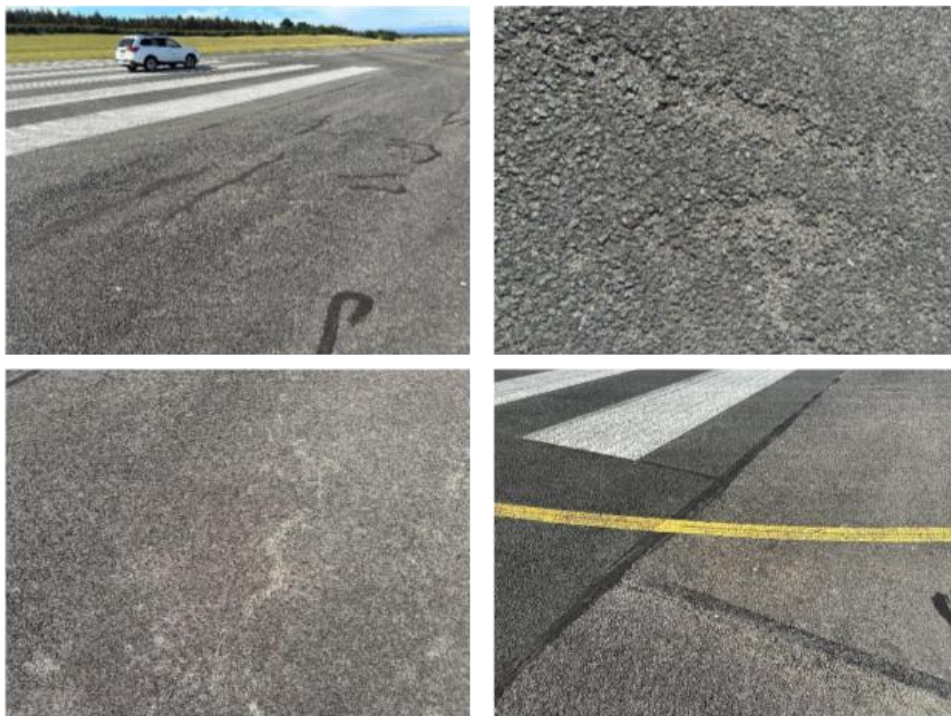
Figure 3-1: Northern Turning Node – Accelerated weathering, white staining, aggregate loss
