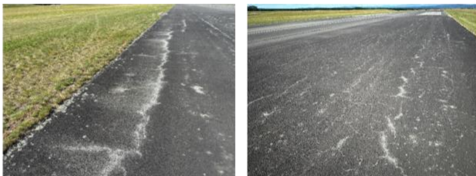
Figure 3-3: Main Runway – Age-related cracking and white staining
