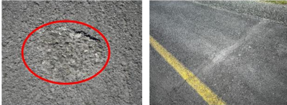
Figure 3-8: Taxiway A – Crocodile cracking, longitudinal/transverse cracking, white staining, debonding
